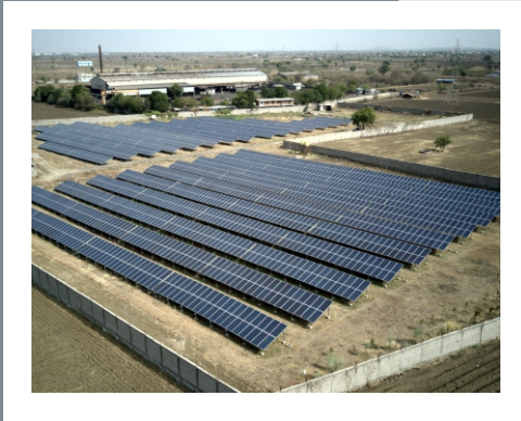
1 Mw Ground Mounted Project
